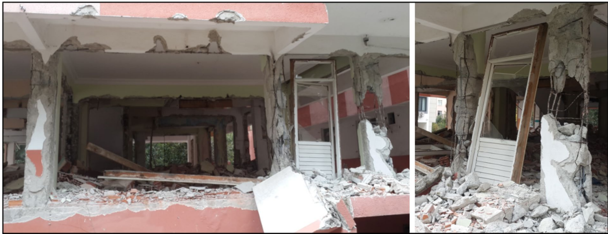
Fig. 9 Two heavily damaged corner columns for HD-I
