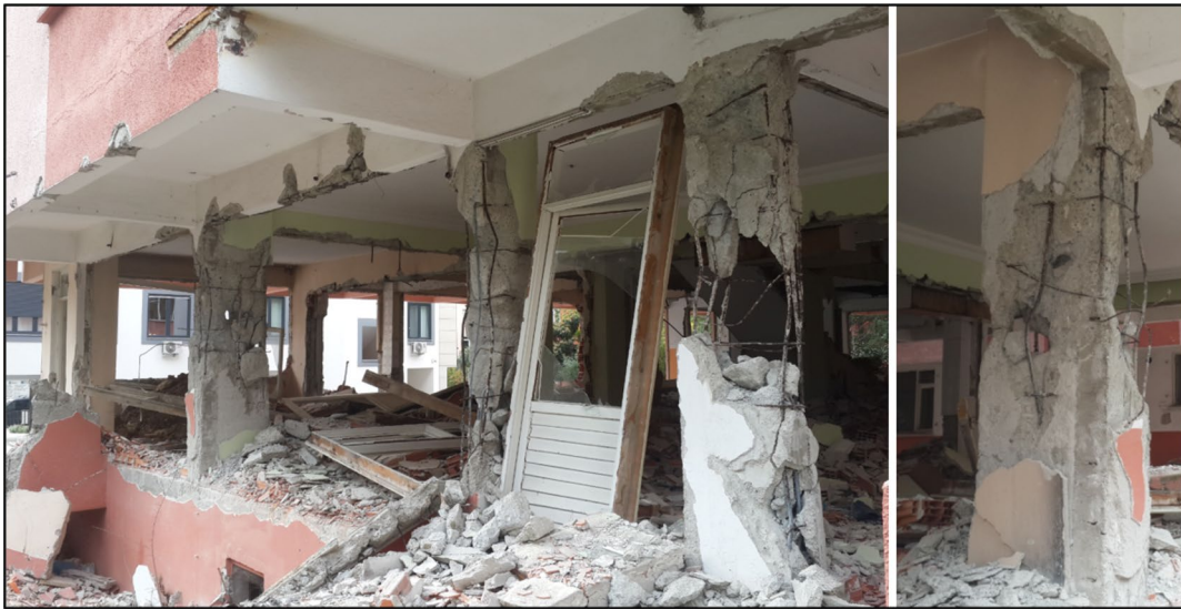
Fig. 11 Heavily damaged three columns for HD-II
