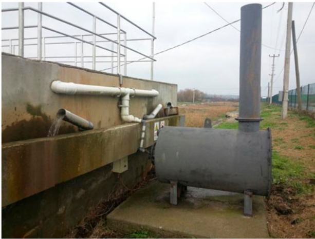
Fig. 2. Gas collection and burning system in anaerobic reactor of Balcik (photo from the system).
